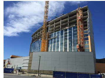
The Southwest Chapter was able to tour the Muckleshoot Casino expansion project last month.
