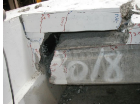
Positive Moment Failure (PMF)
