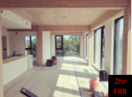
Type IVC - Carbon 12, Portland OR 8-Story wood over 1 Story Concrete <85ft, Exposed Wood 2hr FRR
