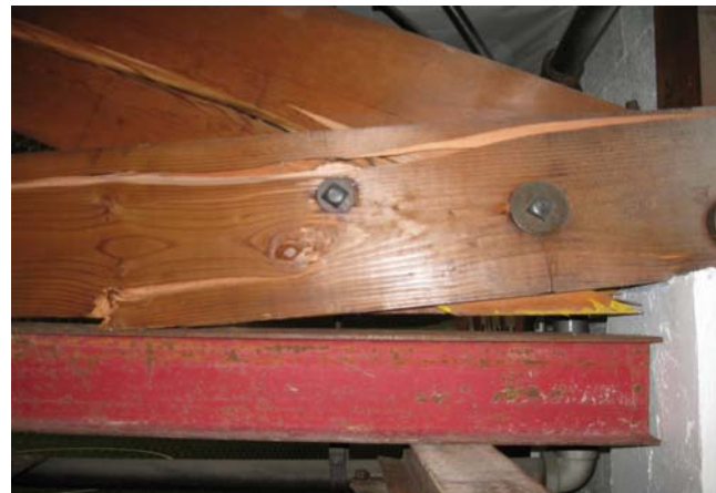
Photo 7: Failed Bowstring Truss Heel Connection
