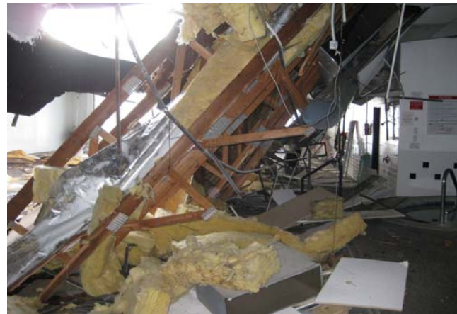
Photo 6: Failed Trusses Over Indoor Pool
