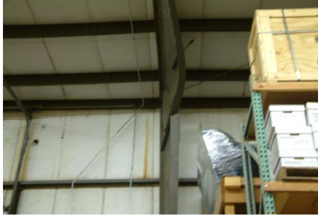
Photo 10: Buckled/Twisted Beam and Column
