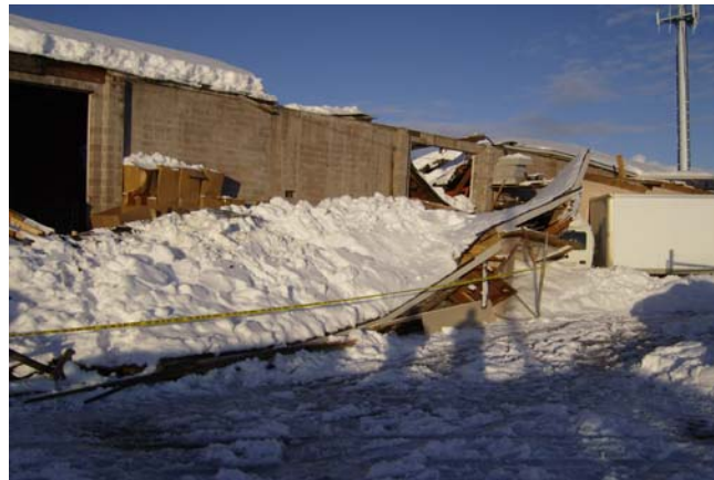
Photo 1: Failed Canopy and Bowstring Truss Roof
