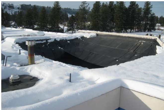
Photo 12: Collapsed Low-Slope Roof
