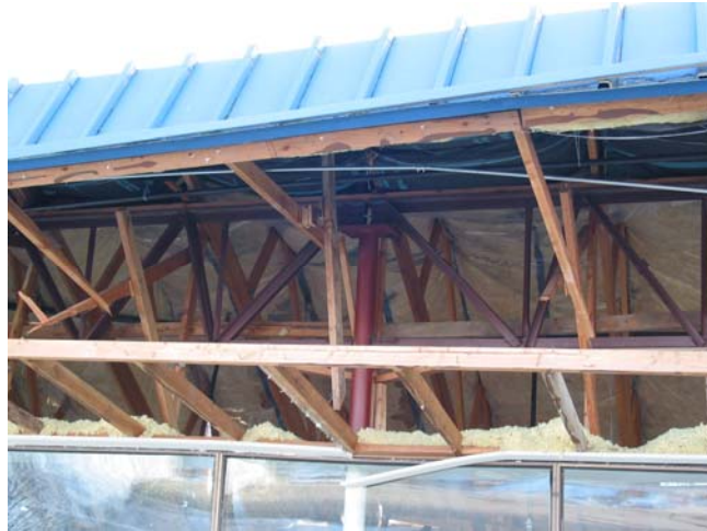
Photo 5: Failed Trusses at Retail Building
