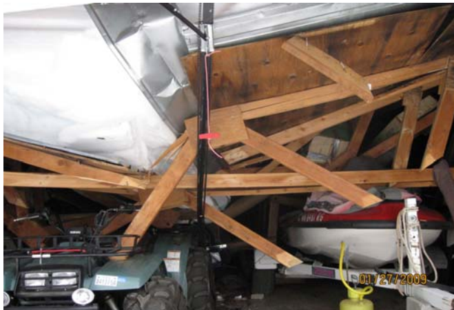
Photo 11: Failed Garage Trusses
