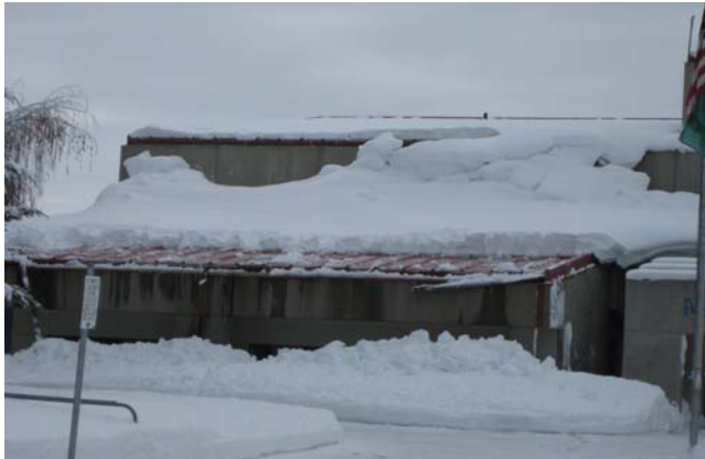
Photo 4: Sliding Snow on Lower Roof
