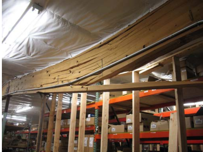
Photo 8: Failed Glue Laminated Beam
